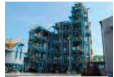
Photo 2 Pressurized, two-stage gasification plant
